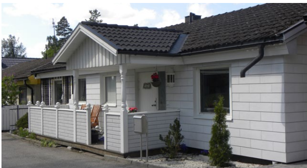
Displaced vertical joints
